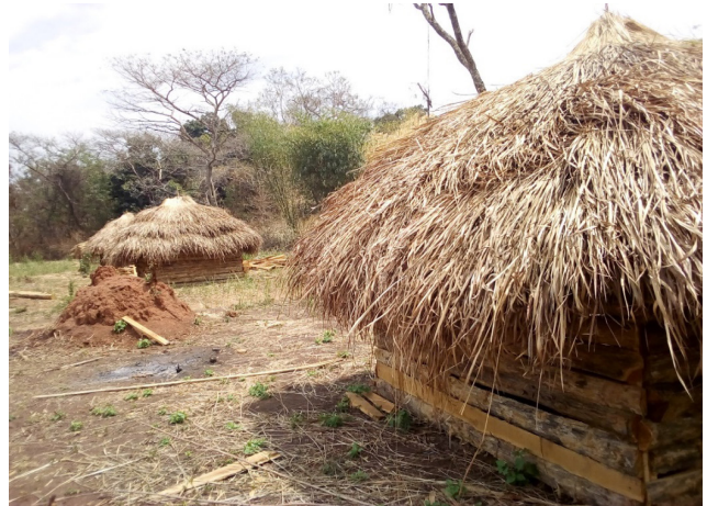
▲ Constructed staff quarters at Bangasu PHCC by the Health Unit Management Committees and the community members.
